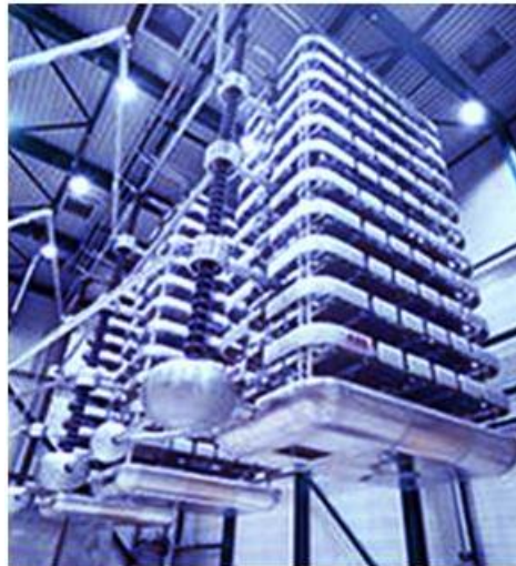
New level UHVDC transmission "Xiangjiaba and Shanghai in China" (7GW, \pm 800 kV, 4200A)
