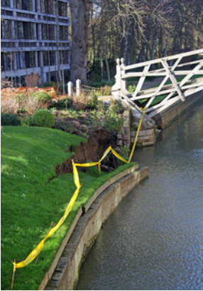
The collapsed river wall. Photo: Dr Jonathan Holmes.
